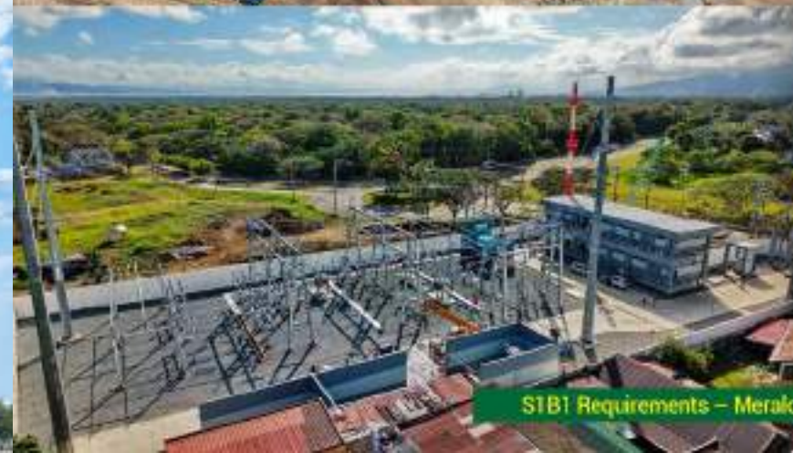
113MWP Binalonan 1 Solar Power Project
